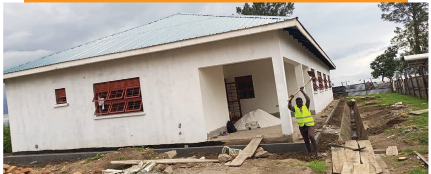
The New NICU Building at Bwera Hospital, a Gift from the Japanese Embassy, Promising a Brighter Future for Preterm Infants.
